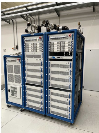
MACHINA 100kW Liquid cooling
